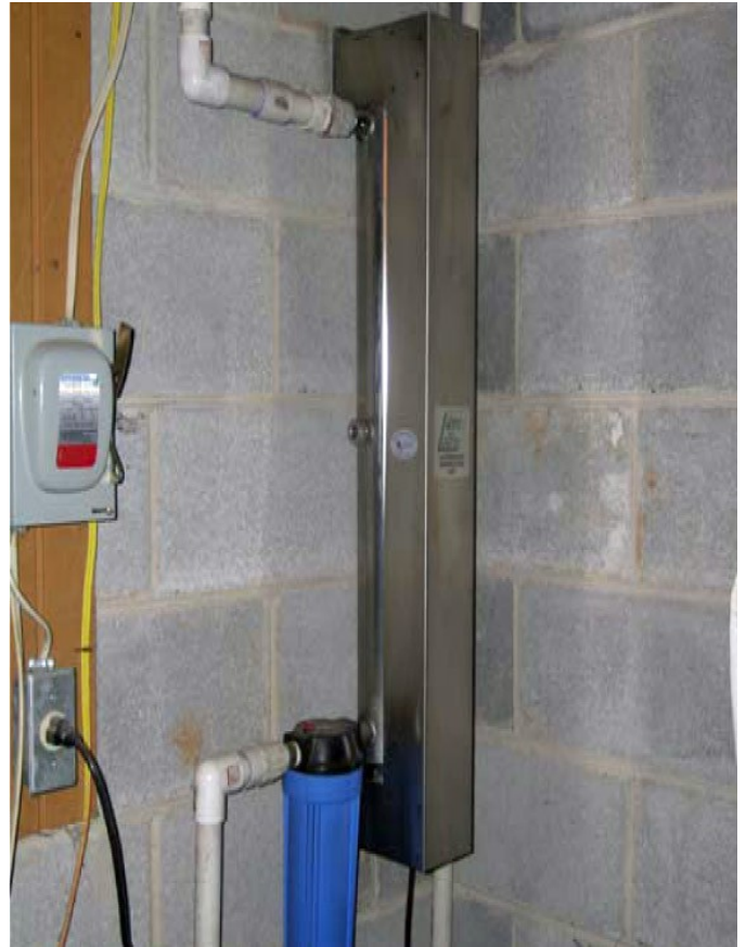
Figure 2. A typical UV light installation with a small canister sediment filter (bottom) ahead of the UV light unit.
